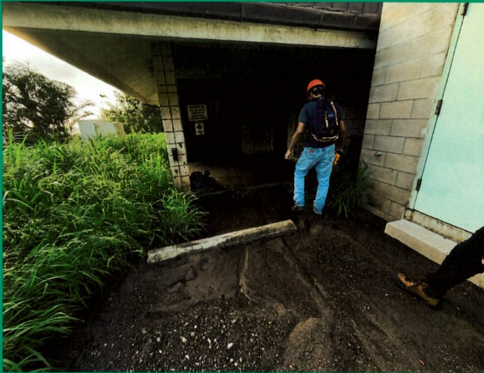
Mud accumulated at the front entrance to the Mākaha Well V control building. HECO transformer can be seen in the background, slightly downhill from the front entrance.
