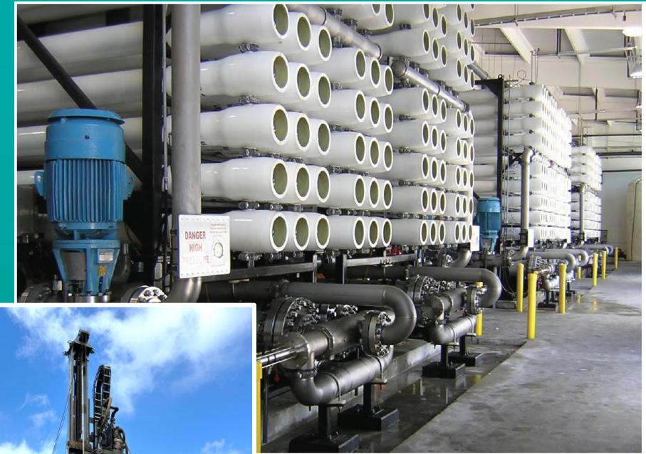
Typical RO treatment facility – Kalaeloa Desalco
