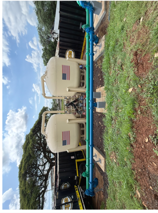
Temporary treatment system at Ka'amilo Wells
