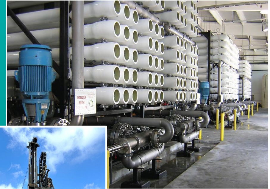
Typical RO treatment facility – Kalaeloa Desalco
