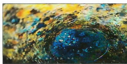
Rust and Corrosion At Top of Water Table
