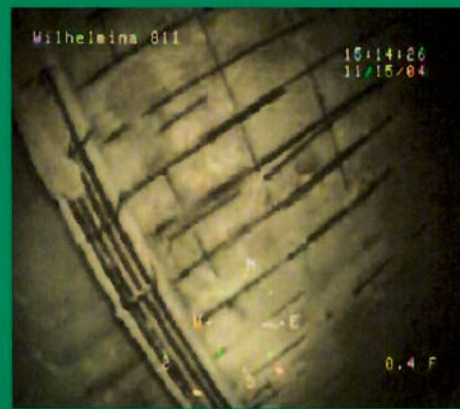
Roof Soffit, roof slab support beams – significant spalling and exposed reinforcing. Insufficient concrete cover and section loss of concrete.
