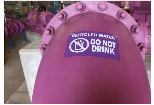
Nonpotable water from the Honouliuli Water Recycling Facility is distributed to users via purple colored pipes.
