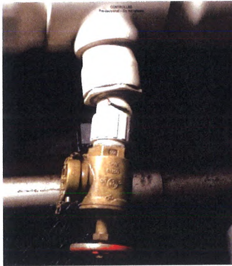
Cracked Low Point Drain
