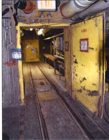
Figure 1: Image of open oil-tight door (foreground) and closed ventilation door on either side of the damaged fire suppression system low point drain valve. [Encl (169)]
