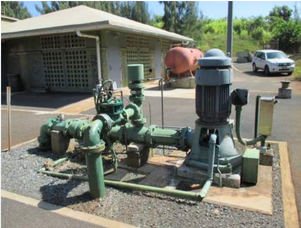
Kahuku Wells Capacity Expansion - To enable BWS to meet its water commitments and sustain system reliability, a 1-million gallon-per-day pump will be added to augment capacity of the existing Kahuku Wells Station, in addition to an emergency generator and building improvements.
