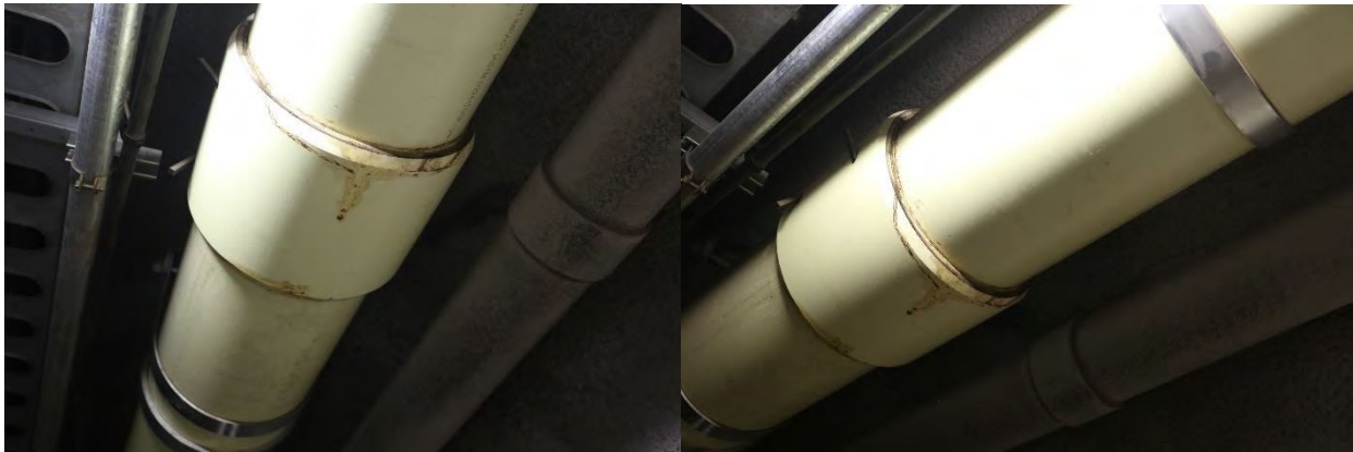
Installed PVC AFFF Retention Line with Joint Seepage
