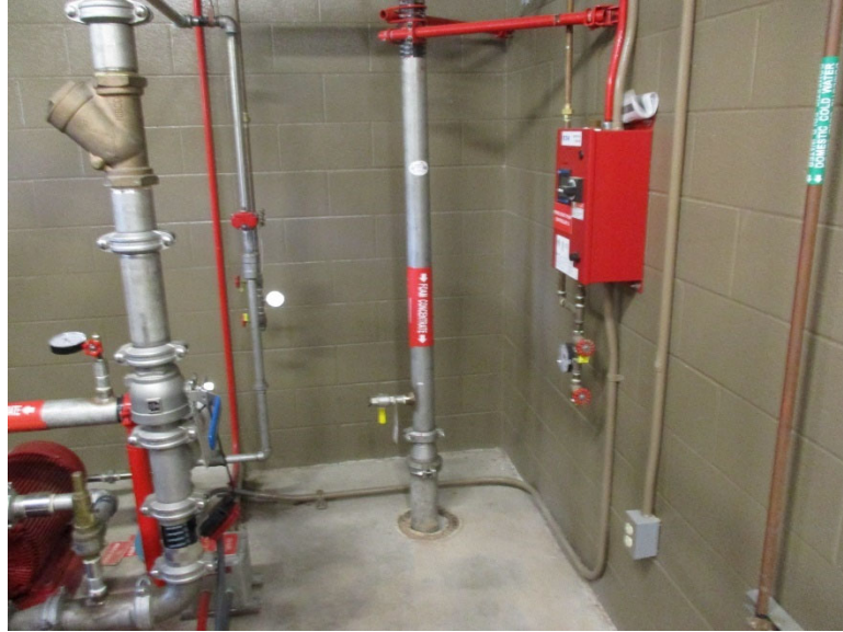
IMG_3054.JPG, taken by author on 6 Dec 2022 – AFFF Concentrate piping existing Building (b) (6)
