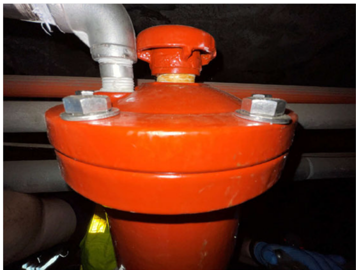
Adit 6 - Air vacuum valve, back view.
