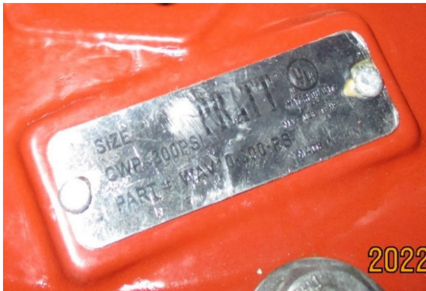
IMG_3158.JPG – Cropped/Enlarged image of Air Vacuum Valve Nameplate
