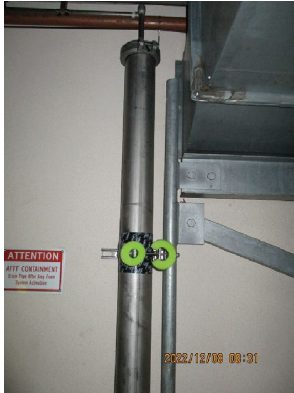
IMG_3139.JPG, taken by author on 8 Dec 2022 – Drain Containment Vessel
