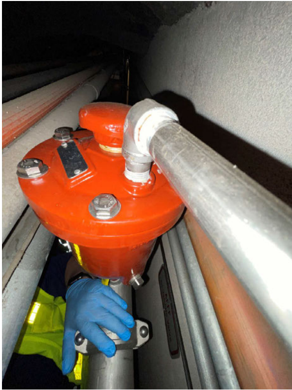
Adit 6 - Air vacuum valve with vent piping connected to flush inlet connection instead of air vent connection (occupied by mushroom)
