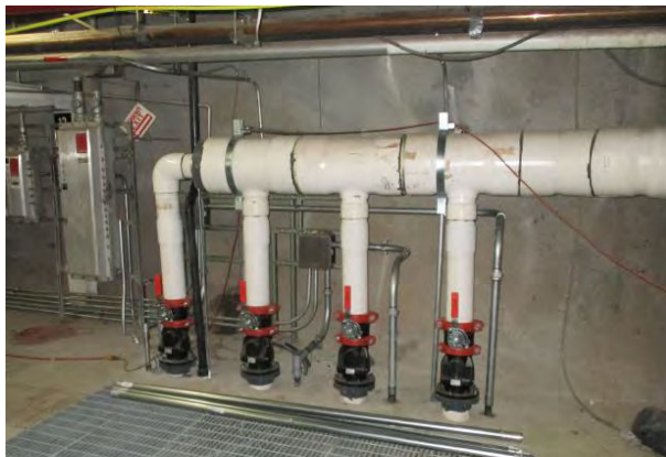
Original AFFF Retention Line Piping in Immediate Area of an AFFF Sump
