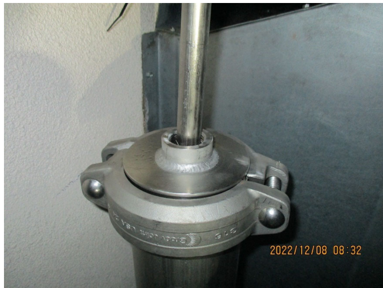
IMG_3143.JPG, taken by author on 8 Dec 2022 – Drain piping connection to drain containment vessel
