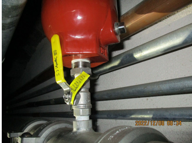
IMG_3150.JPG, taken by author on 8 Dec 2022 – Connection of Air Vacuum Valve to concentrate piping
