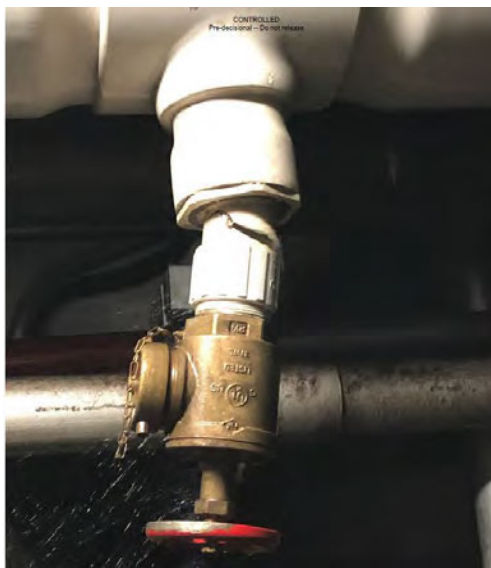
Cracked Low Point Drain
